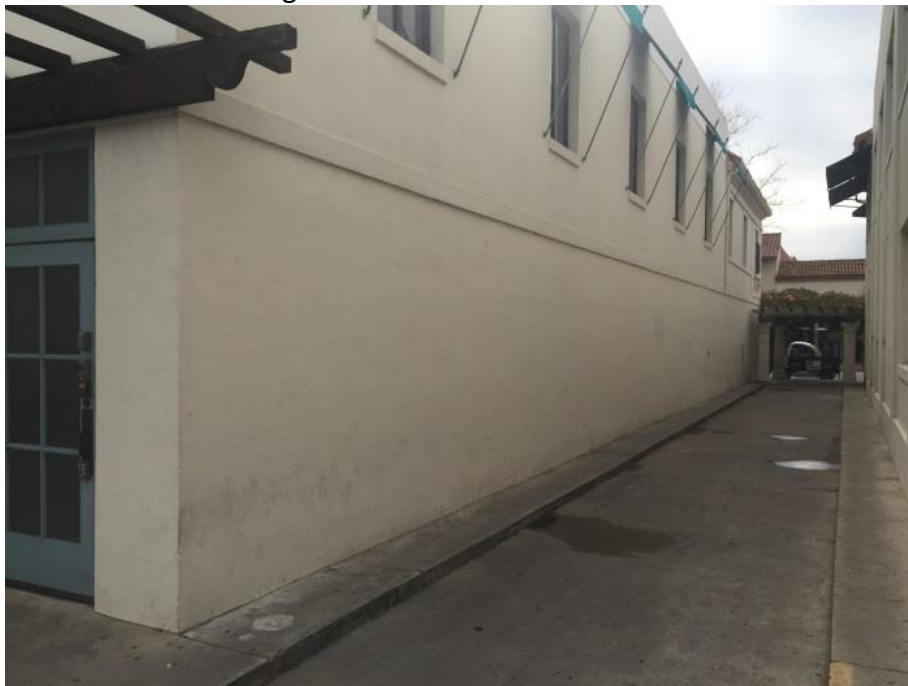
Image #2 - from the outside parking area behind the Granada Garage looking west towards State Street with the North facing wall of 1214 State Street visible
